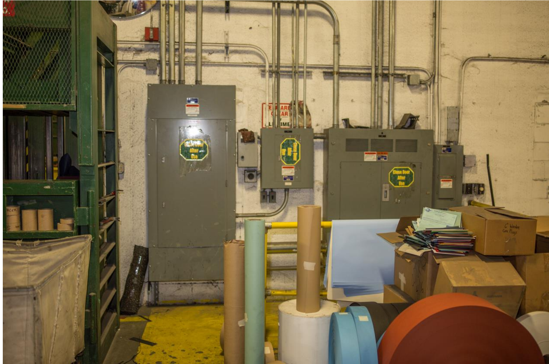
Interior Electrical Panel
