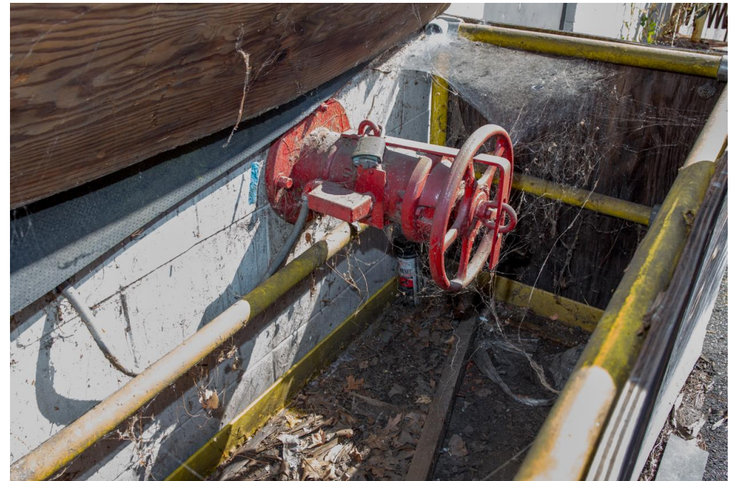
System 2 - South Side of Building
